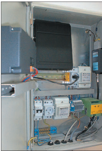
Electricity cabinet in the SW 110 group centre Goleszowska street
